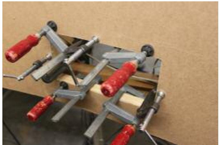
After the panel hole has been cut into the fascia, 1x1 pine strips are clamped and glued to the backside.
