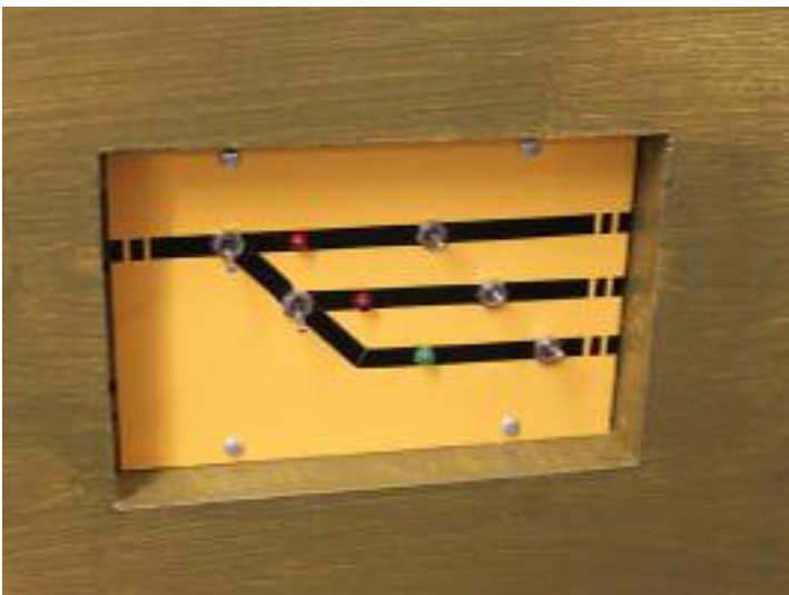
Here is a finished and installed panel in place. Note how the toggle switches do not extend past the edge of the fascia.
