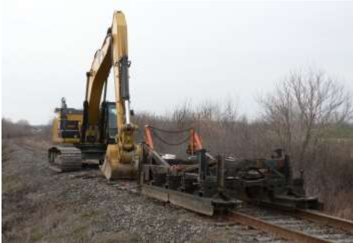
Top: The other tool used in the removal of the rails – a backhoe and a custom designed sled aiding in the pulling of the spikes.
