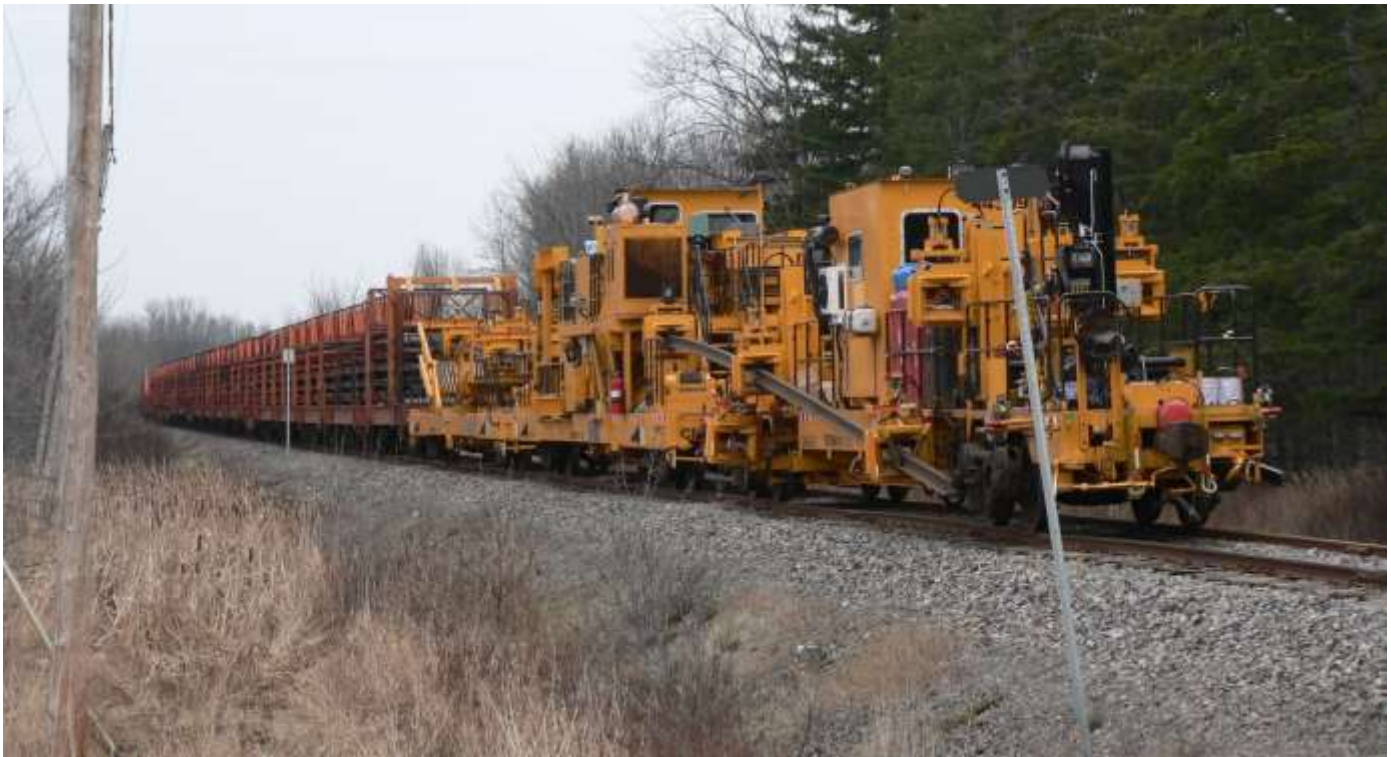
Top: Rail removal train parked on the Renfrew subdivision on the weekend after completing the removal of the tracks on the Beachburg sub between the Ottawa river and Renfrew Junction.
